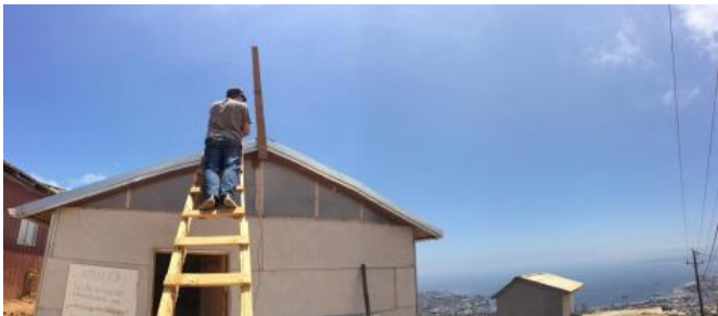
Fig. 32. Ignacio Nieto, installing a mesh router. Cerro Mariposa (Butterfly Hill), Valparaiso. Photo: Mauricio Roman.
